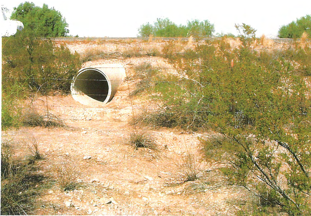
Figure 6: A culvert seen from the extreme northwest portion of the Parcel. Flows from the northern slopes of the Parcel are channeled here and other culverts under I-8 off property, which dissipate to sheet flow.
