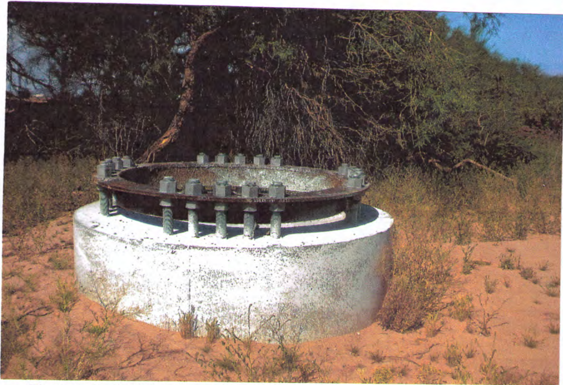
Photographs #7 & #8 - Views of one of three utility related foundations on north parcels -
