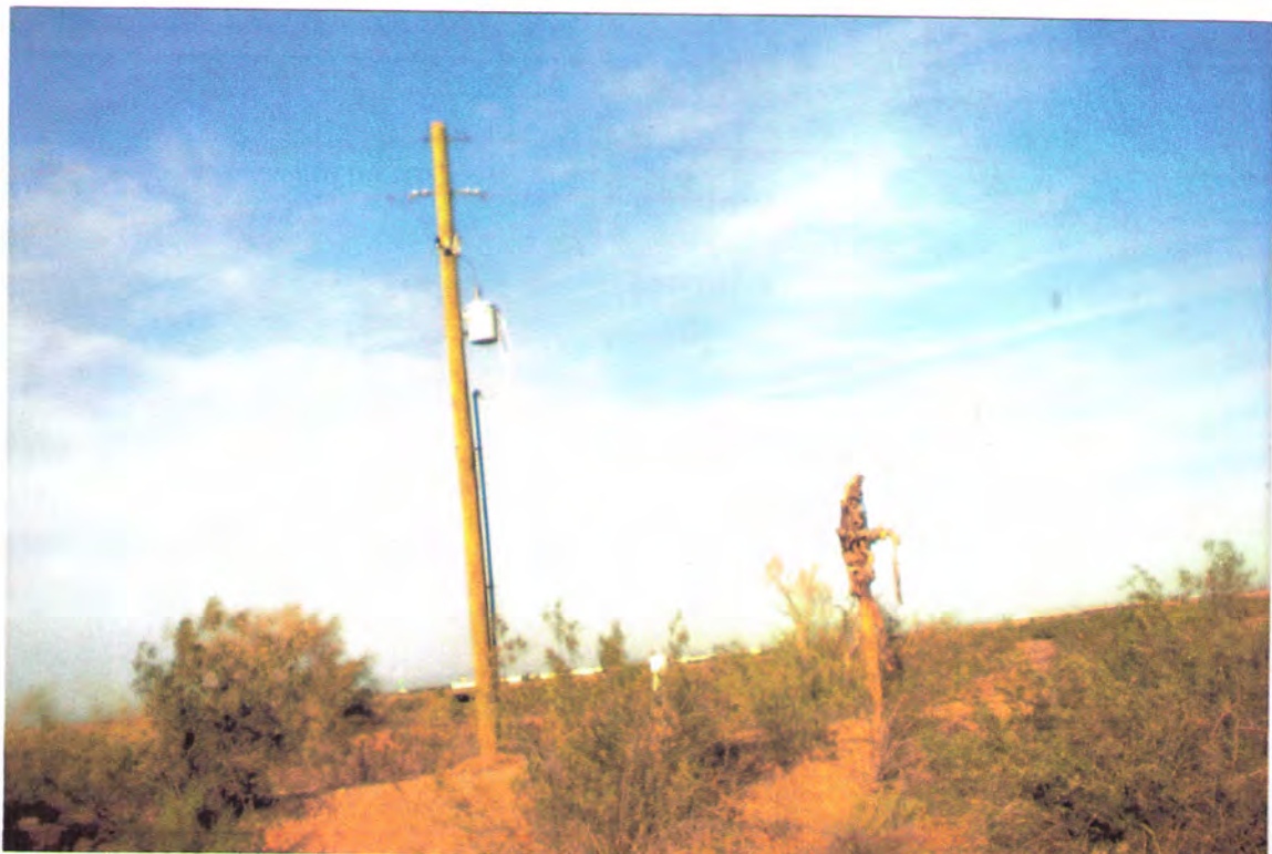
Photograph #12 - View of pole-mounted transformer located along northern site vicinity of south parcels -
