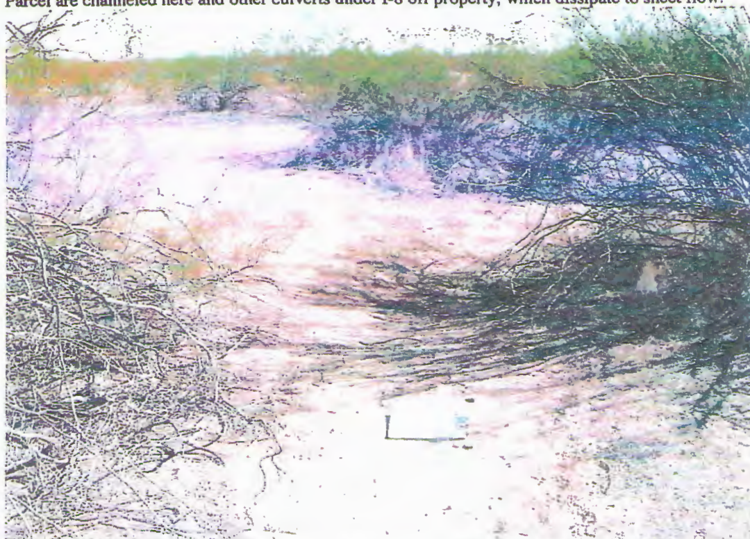
Figure 7: Resulting offsite dispersion and dissipation of flows from the culvert in Figure 6.
